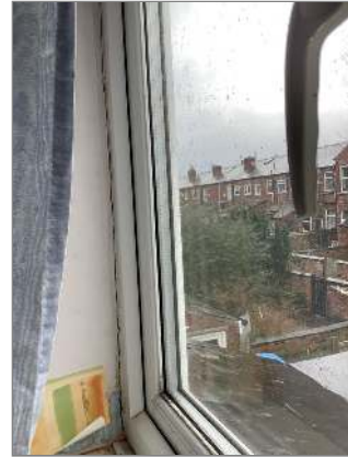
Photo - 49 Gaps between rear bedroom window frame and the wall
