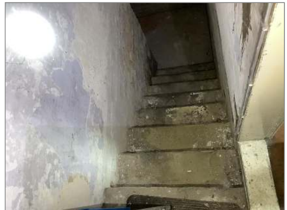
Photo - 165 Solid staircase no handrail
