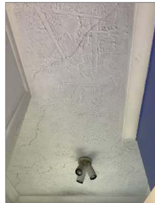
Photo - 83 Cracks to textured coating ceiling to bathroom
