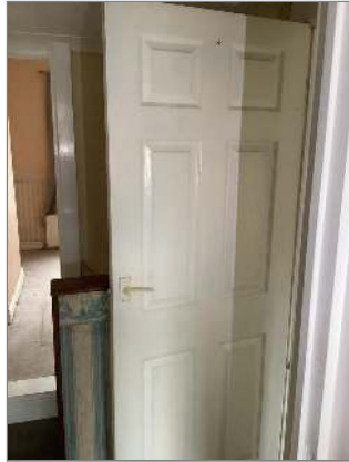
Photo - 148 Creaking rear bedroom door
