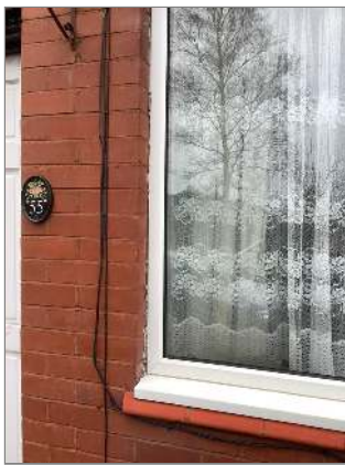
Photo - 44 Gaps to sealant to the front lounge
