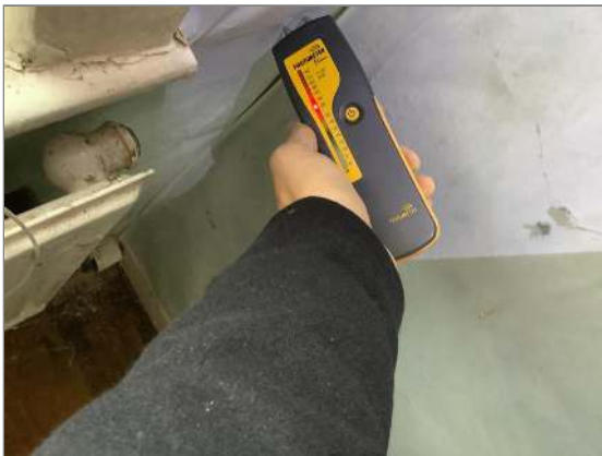
Photo - 109 Likely defective plaster to the rear wall near party wall
