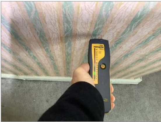
Photo - 128 Front bedroom
