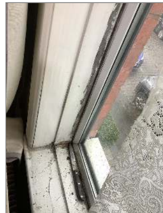
Photo - 47 Gaps between front bedroom window frame and timber sub-frame
