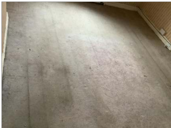
Photo - 116 Carpet with creaking and bouncing floorboard to front bedroom
