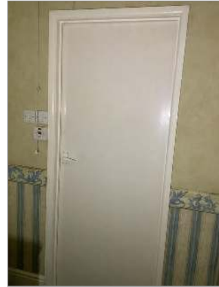
Photo - 149 Bathroom door panel rub against door frame
