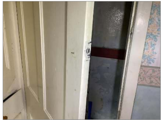
Photo - 155 Defective lock to the basement door
