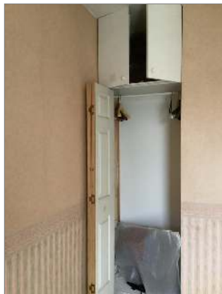
Photo - 140 Stiff doors to the upper cabinet
