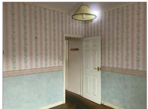
Photo - 106 Solid walls with wallpaper in the rear lounge
