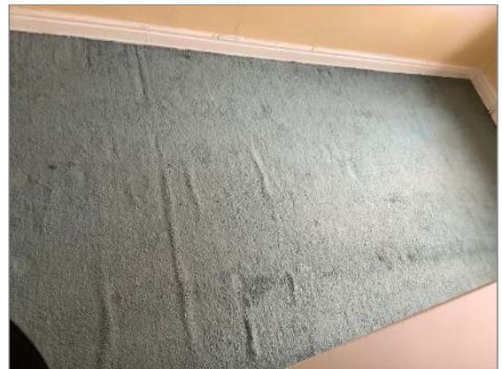
Photo - 117 Bouncing floorboard and aged carpet to rear bedroom
