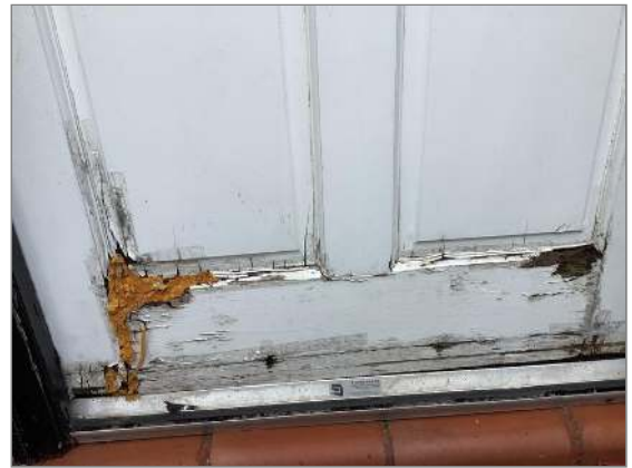
Photo - 58 Defective and rotted timber door
