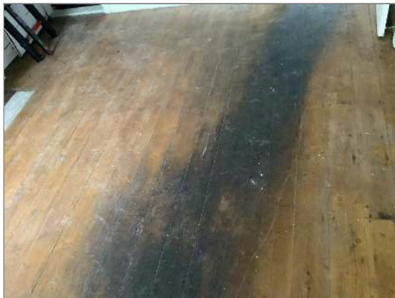
Photo - 122 Minor vibration to the timber floor board in rear lounge
