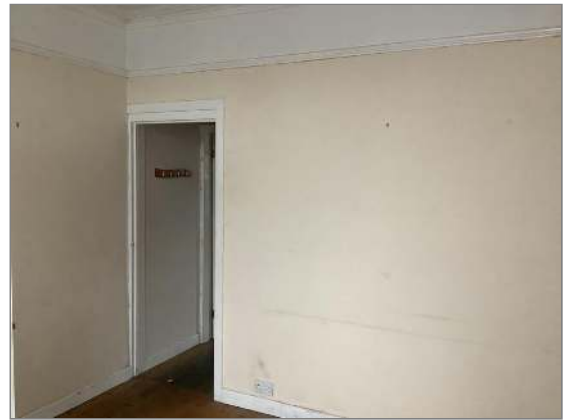
Photo - 102 Painted plaster to solid walls of front lounge
