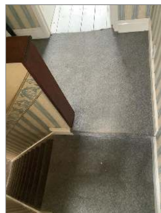
Photo - 119 Bouncing and creaking landing
