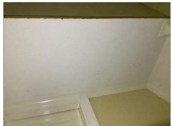
Photo - 85 Textured coating to lowered landing ceiling
