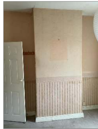
Photo - 129 Front bedroom
