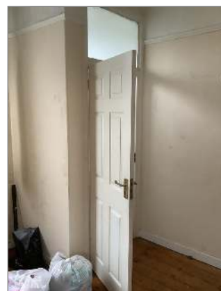
Photo - 153 Vestibule door panel rub against door frame
