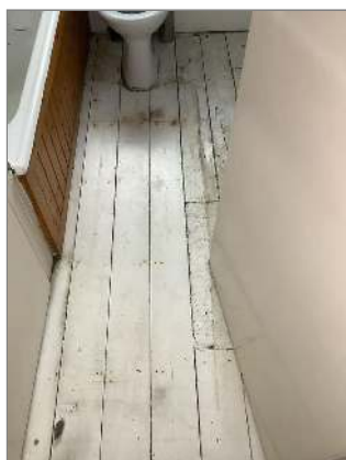
Photo - 118 Timber floorboard bouncing near WC
