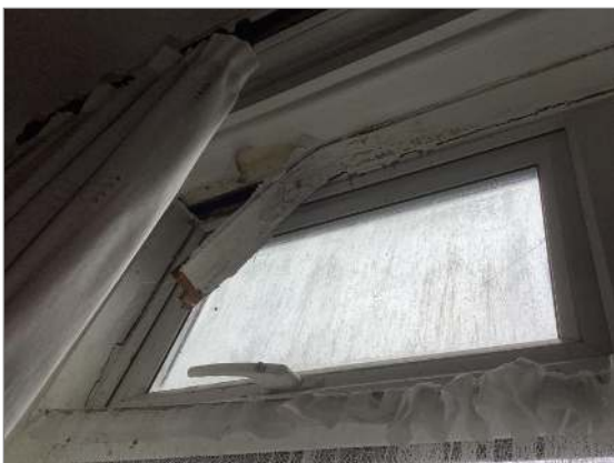
Photo - 52 Detached and rotted timber frame to the front lounge window
