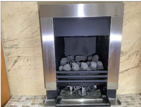
Photo - 136 Gas fire to front lounge
