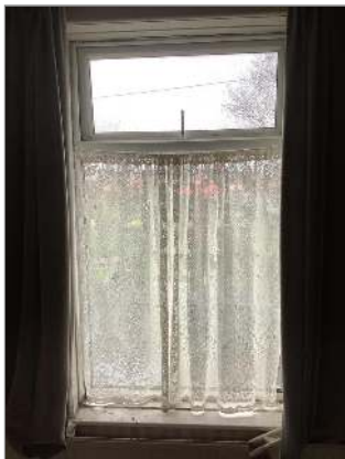
Photo - 46 UPVC double glazed window without safety mark to low level glazing
