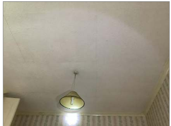
Photo - 89 Rear lounge with hairline crack to textured coating
