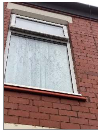
Photo - 45 Gaps to sealant to the front bedroom
