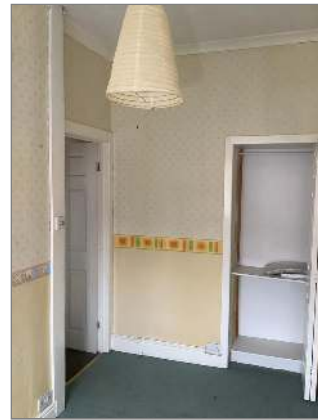
Photo - 96 Wallpaper to stud wall and solid wall in the rear bedroom
